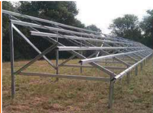
Solar Power Plant Structure
